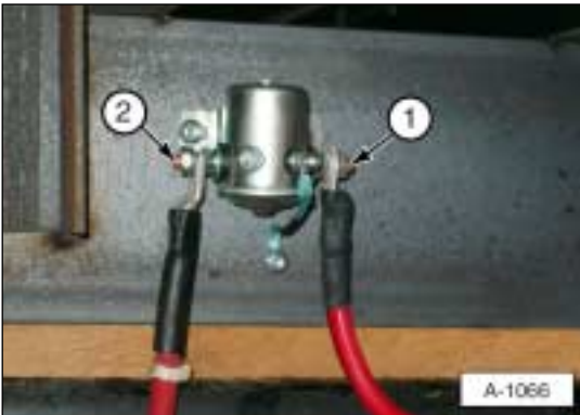
Power cut-off solenoid.
