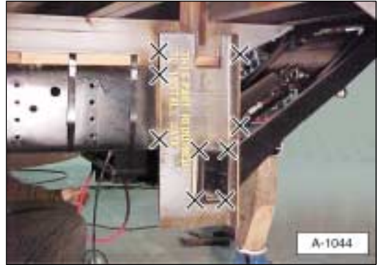
Illustration 12. Put mounting plates into position. Put 3/8" fillet by 1 inch long tack welds at locations marked "X".
