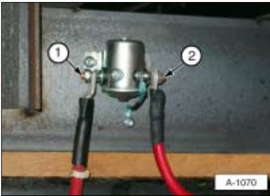
Illustration 9. Cut-off solenoid installed between battery and fuse assembly.
